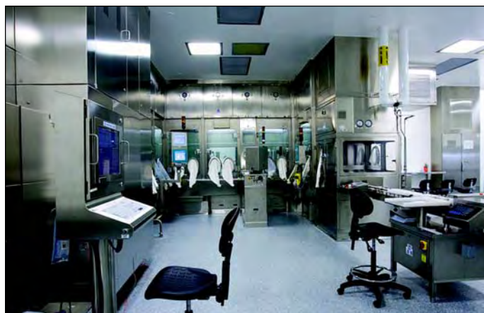
Continuous process isolated fill line.
