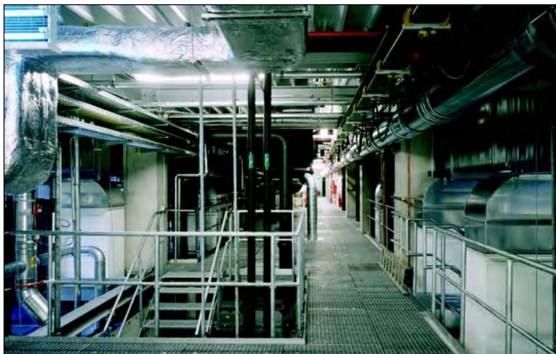
Technical maintenance area adjacent to production rooms.
